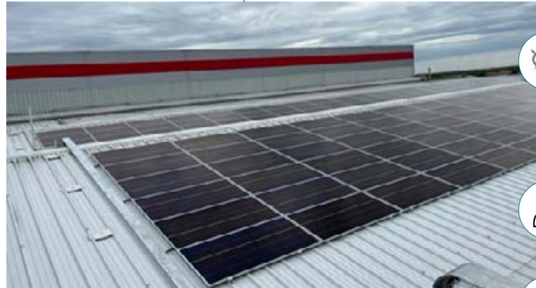
Bertolaso photovoltaic panels
